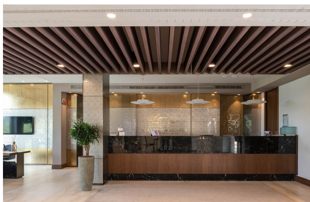
Fig. 2 Acoustic ceiling treatment in the reception area of Palazzo di Varignana (source: Caruso Acoustic [19]).
