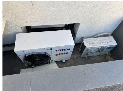
Fig. 3 Noise sources below the ground floor level
