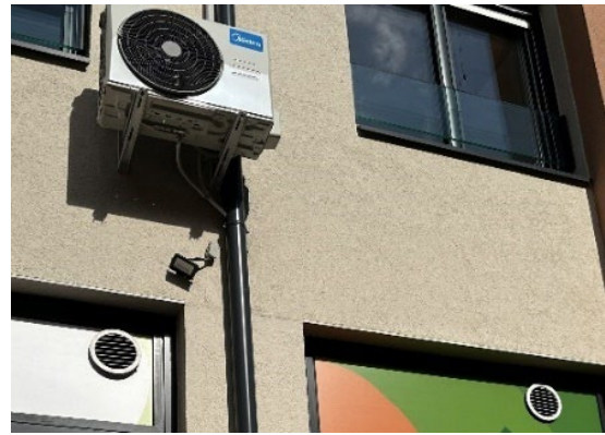
Fig. 6 Exhaust bars below the apartment
