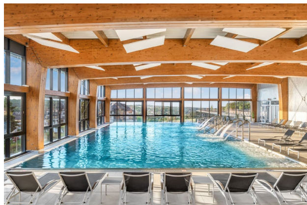
Fig. 3 Suspended ceiling elements in an indoor pool hall, Fruške Terme (source: Eventlin [20]).
